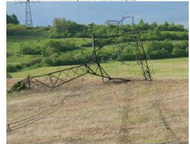
Figure 1-4 Transverse cascade of five 400-kV towers due to a May 2006 HIW storm in Czech Republic. (Photo: P. Froněk)
