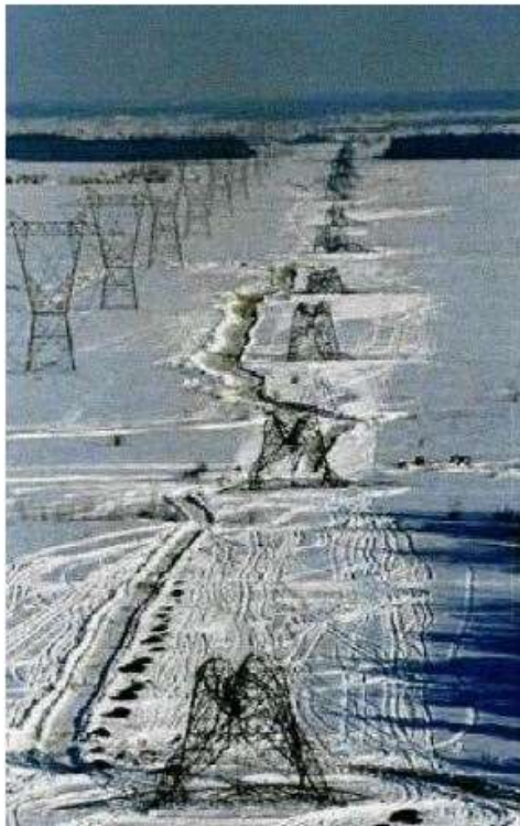
Figure 1-1 Longitudinal cascade on a 735 kV line in Canada during the Great Ice Storm of January 1998. (Photo: B. Breault, La Presse )
